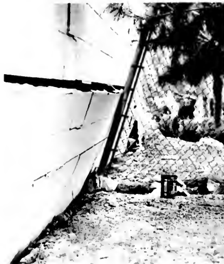
Photo 14. Damage due to ground surface shortening in the Arroyo light industrial tract. E. G. Zacher photo.
